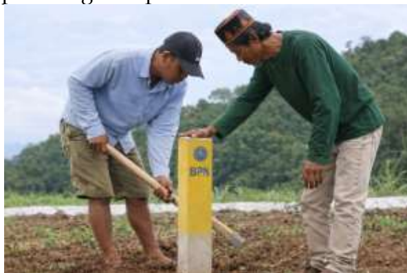
Figure 2. Community Participation in Land Boundary Marker Installation as Part of Systematic Land Registration
